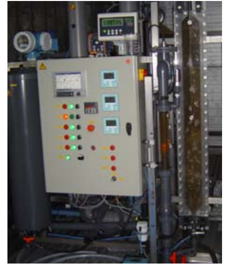
De proefinstallatie OMBR / The pilot plant OMBR
