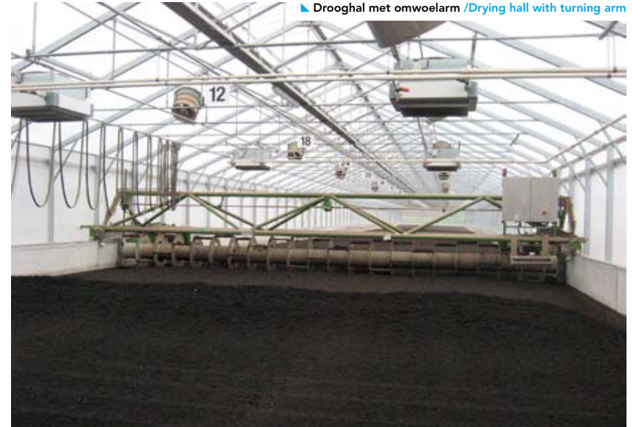
▶ Drooghal met omwoelarm /Drying hall with turning arm
